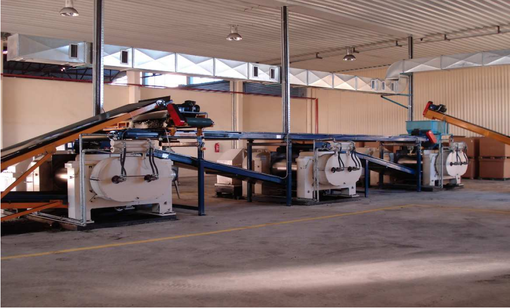
Fig.1: Illustration of the three de-vulcanizing roller – mills with all the necessary auxiliaries, roller mill cooling system etc.
